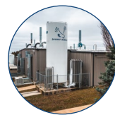
Chiller/Tower replaced January 2022
